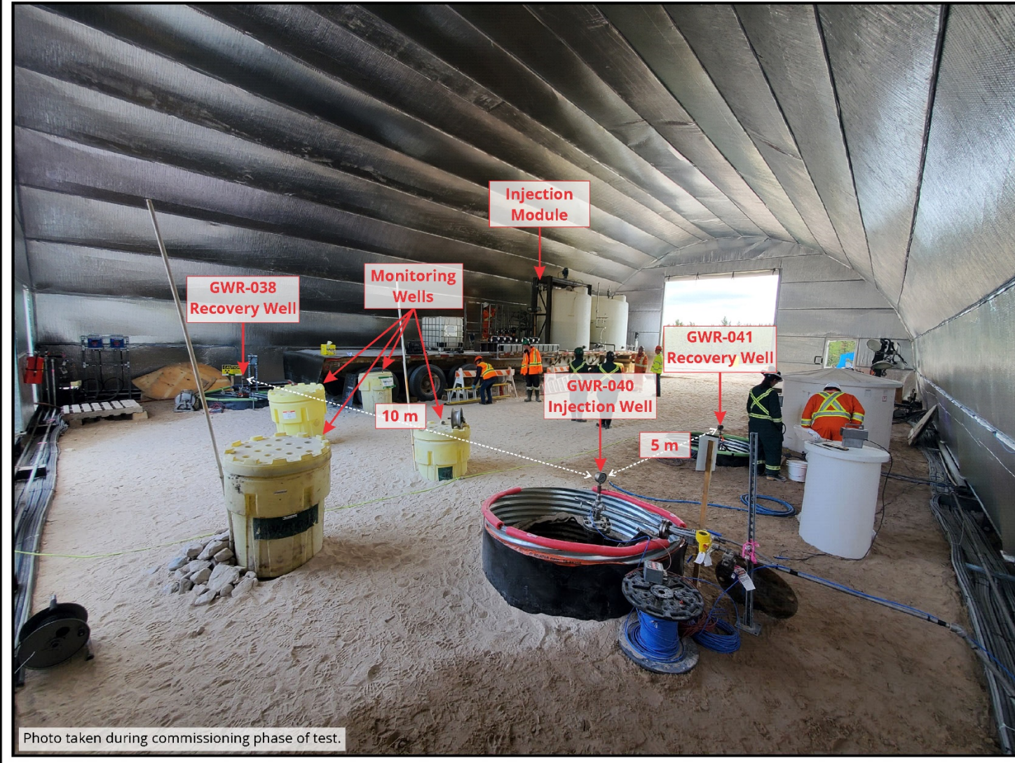
Figure 2: Phoenix – Feasibility Field Test Wells and Injection Module
